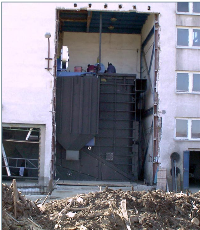
The photographs depict installation of a new biomass boiler in Třebíč's heating plant with an output of 3 MWts that have been serving straight since 2002 (author the TTS company).
